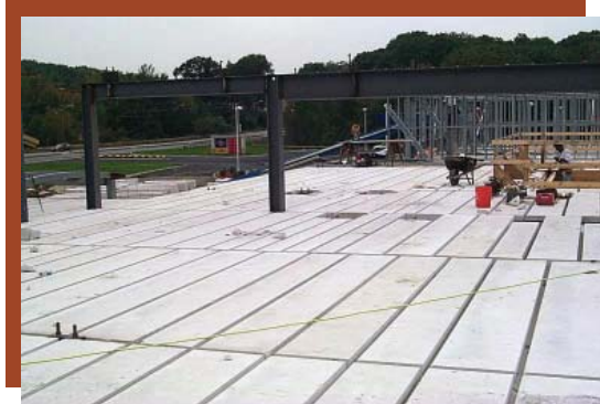
Marriott Hotel, Lincoln, RI: AAC Floor Panels Supported on Light Gauge Metal and Steel Framing (Photo by Dewberry)
