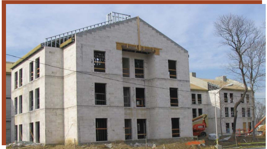
SUNY at Stony Brook Graduate Apartments: AAC Masonry Walls and Precast Hollow Core Floors. (Photo by Dewberry)
